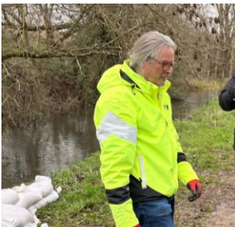
Barry working with volunteers to tackle a breach in the river bank
